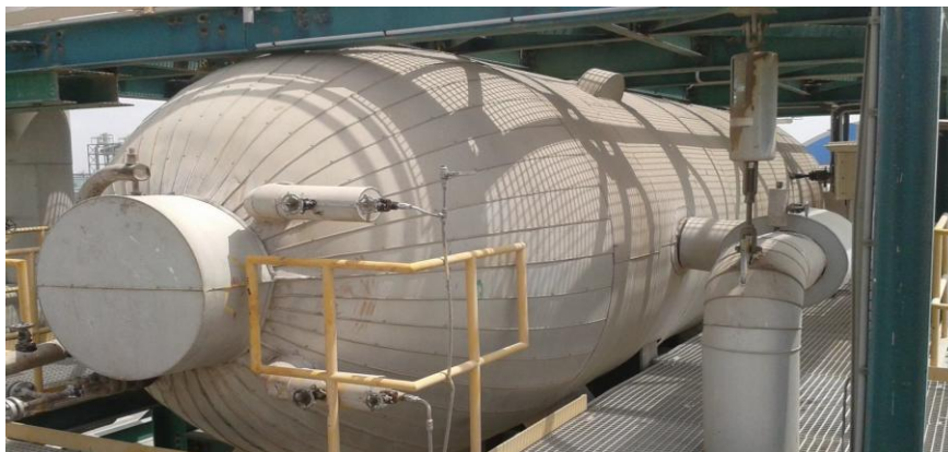
Figure I.8 :Ballon de chaudière. [2]
