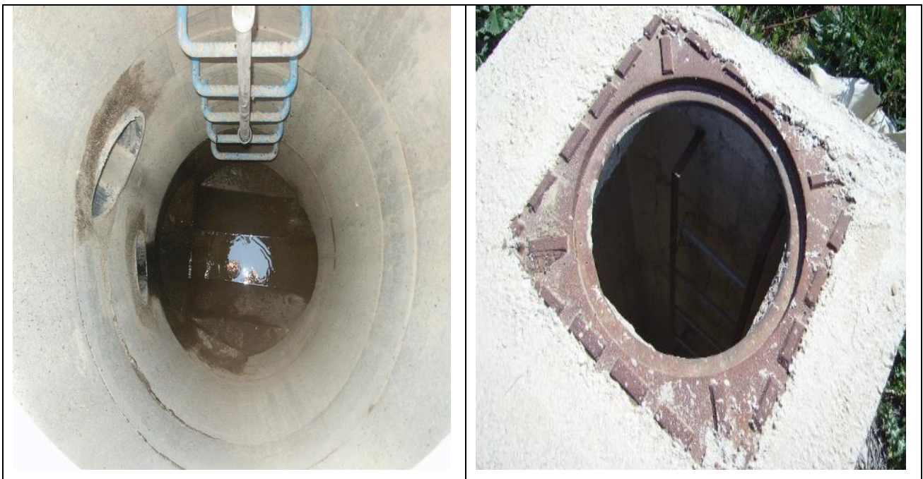
Figure V.5: Regard de visite
