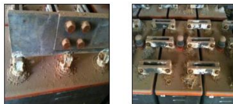
Figure 5. Battery degraded (station of MELOUKA).
