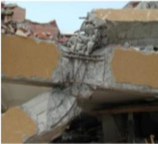
Figure II. 7 : Rupture en zone nodale([32])
