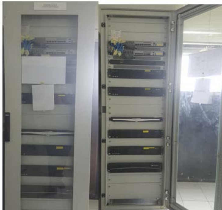
Figure 3.8-Armoire SCADA Terminal Arrivé Bejaia.
