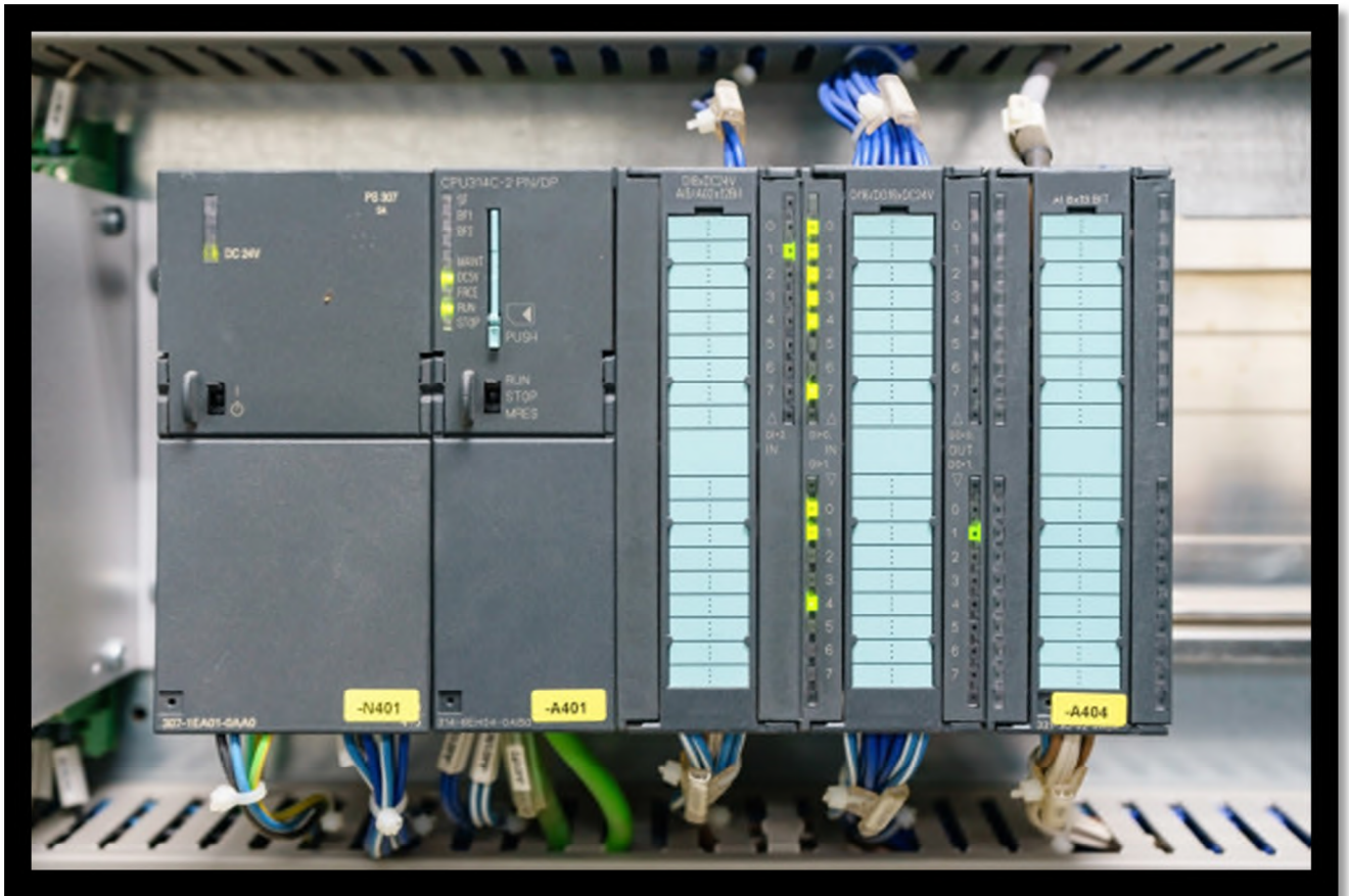
Figure II.1 : Automate Programmable Industriel SIEMENS
