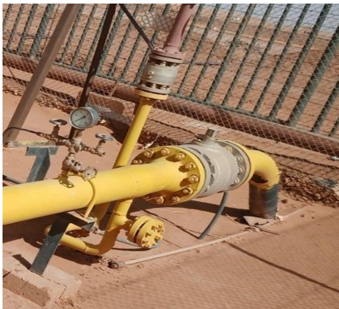
Figure II.9 : Vanne HV-1(photo prise sur site)
