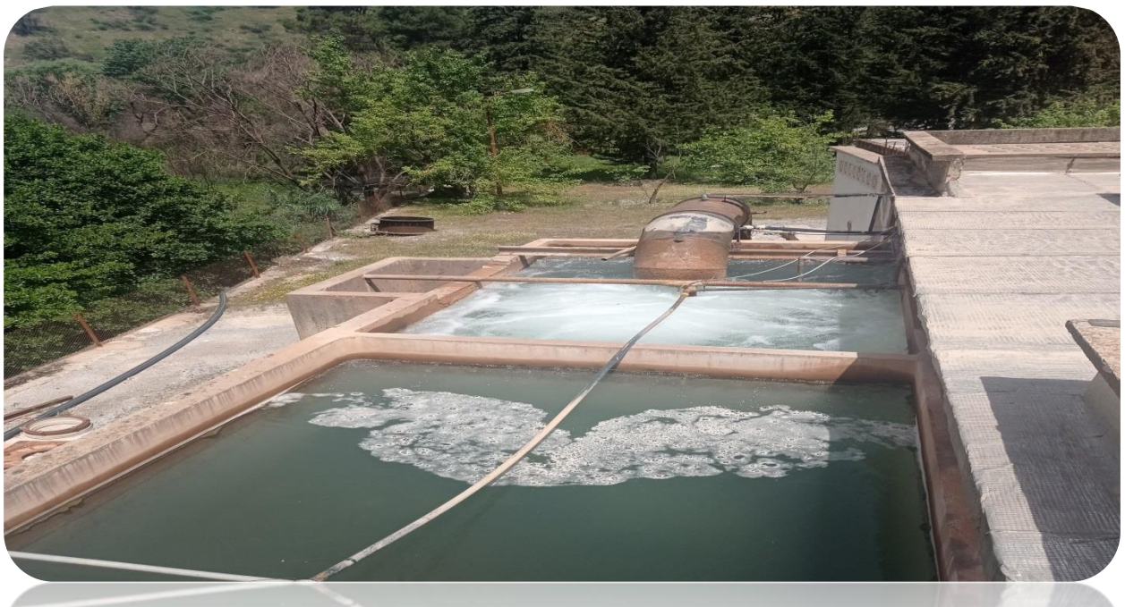
Figure (III.12) : Bassin de coagulation.
