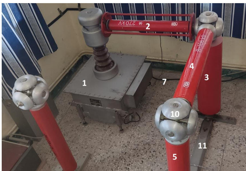
Figure II.7 : Photo de la source haute tension
