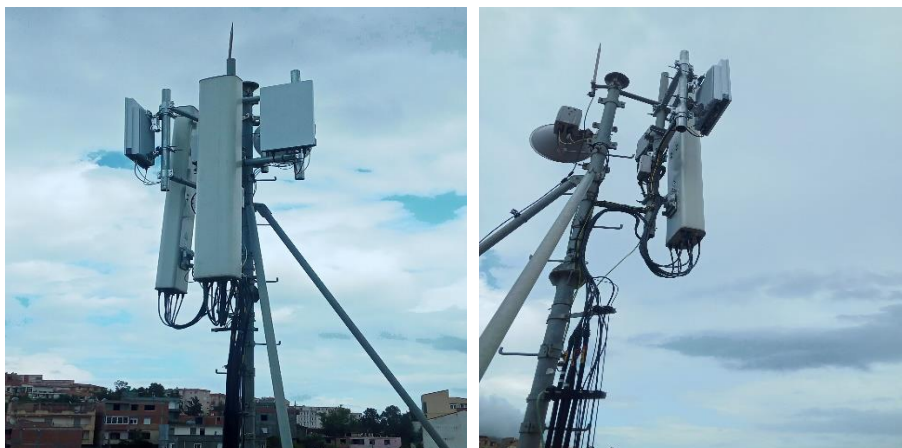
Figure.III.25: Installation de Massive MIMO.
