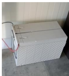
Figure 2-23 : Batteries de secours
