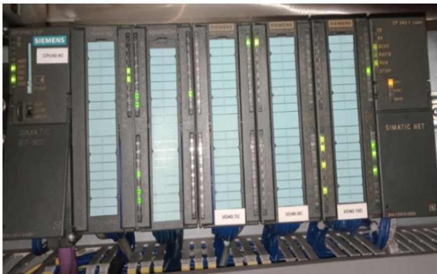
Figure 3.1 : Automate programmable industriel
