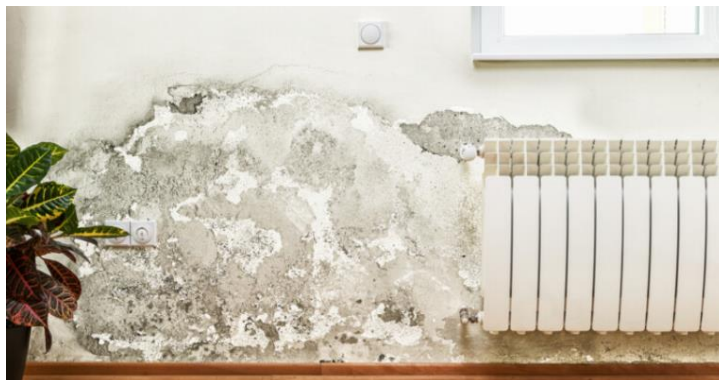
Figure 1.13 : Effect of humidity on walls. (Source: https://dampproofingbournemouth.com , 2023)
