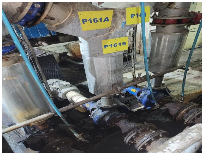
Figure III.6: Pompe centrifuge P161A
