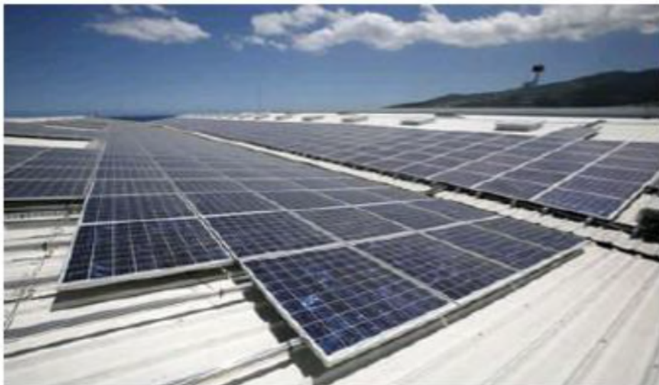
Figure II.6 Panneaux Solaires Photovoltaïque
