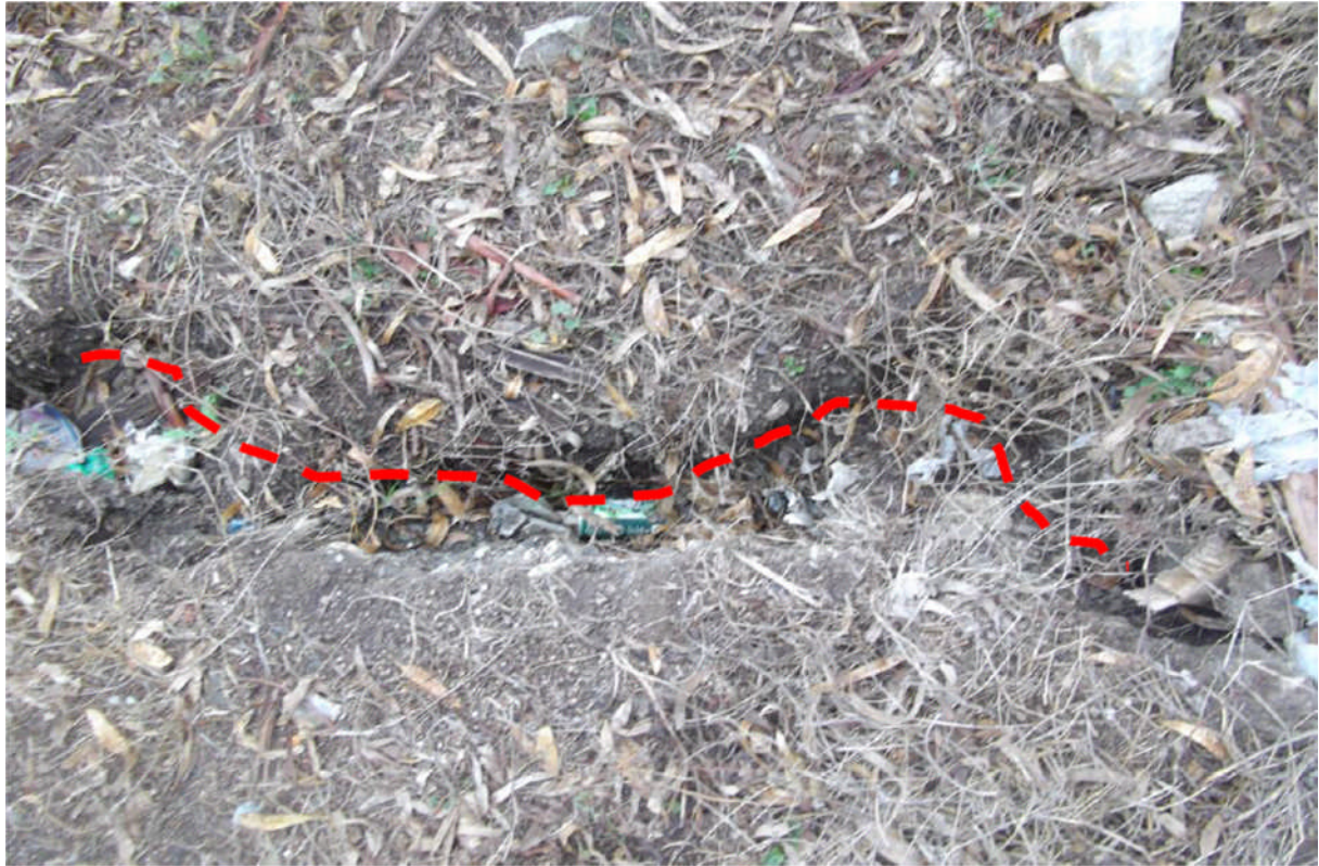
Figure I-9 : Fissures de traction [16].
