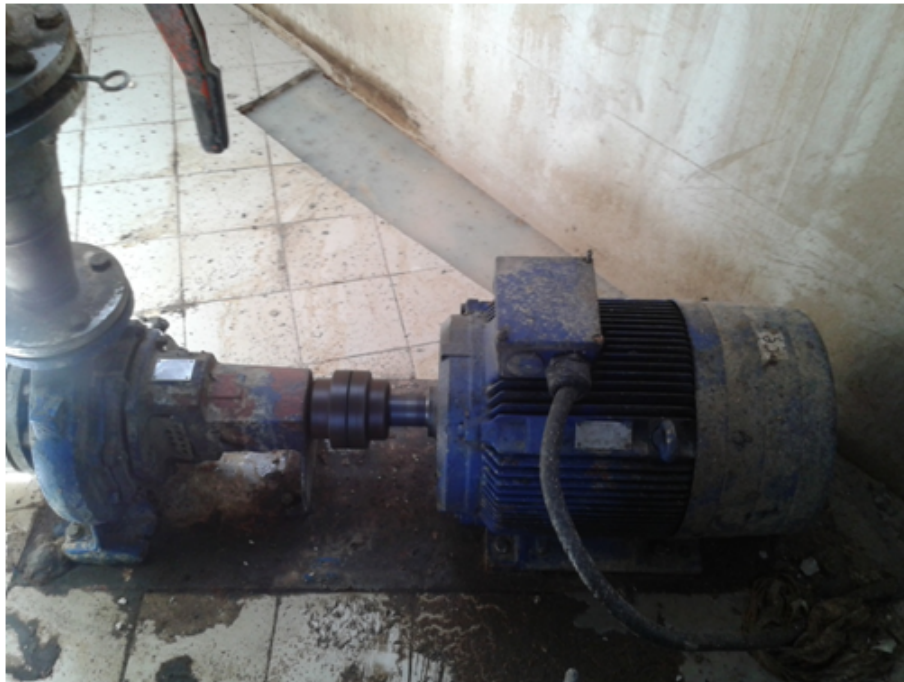
FIGURE 1.3 – la pompe centrifuge
