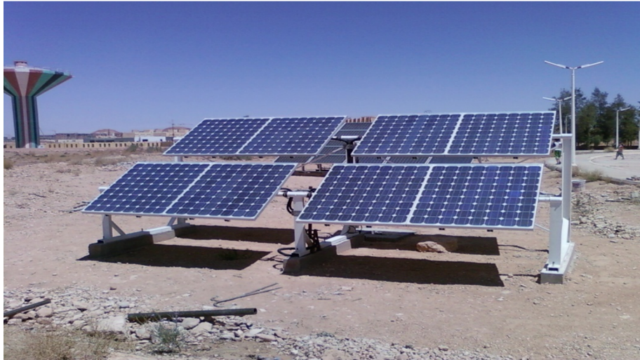
Figure (I.22): Panneaux solaires
