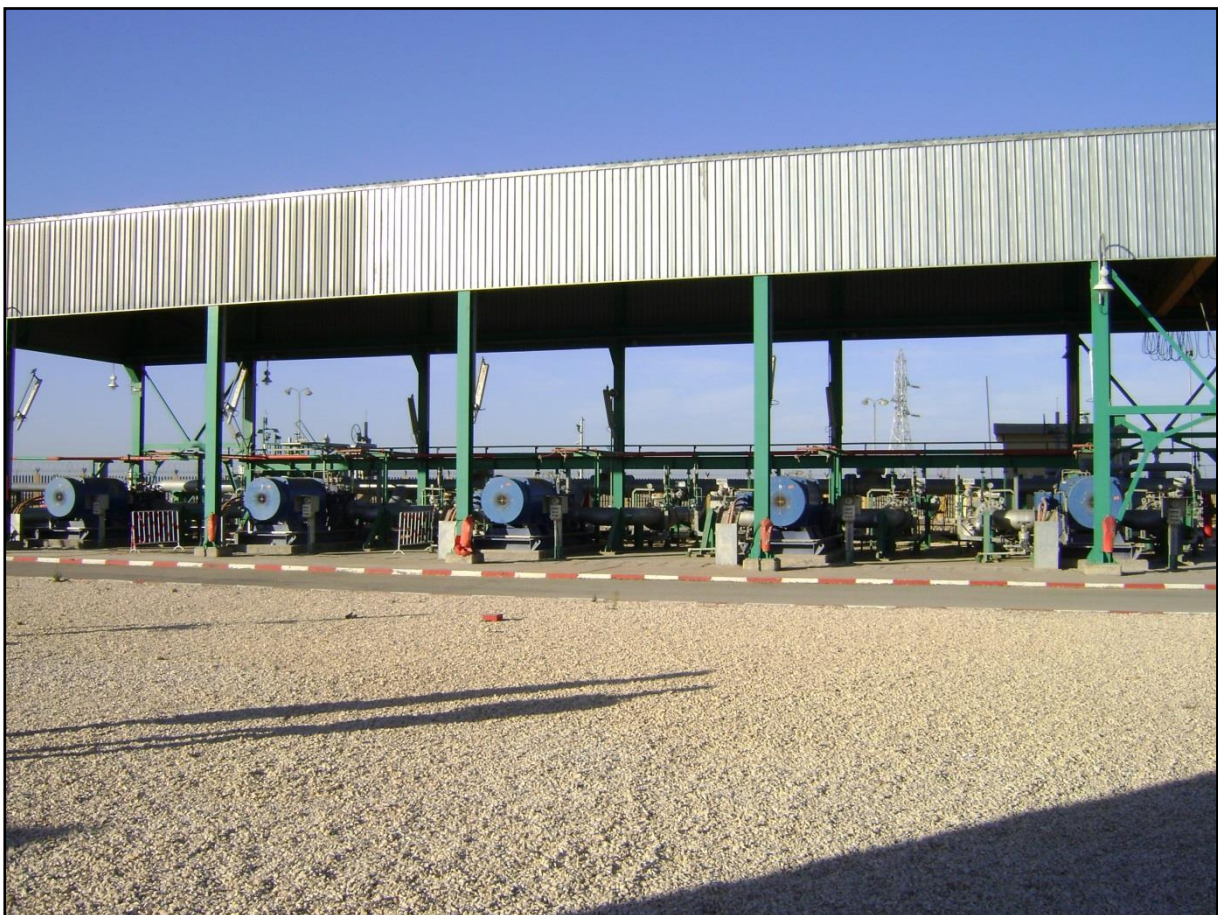
Figure V.1. Station de pompage (D.RG.Biskra)
