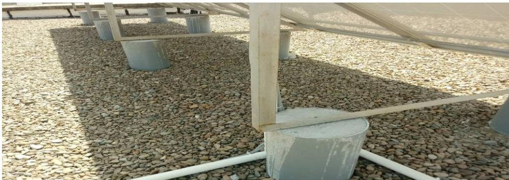
Figure III.11 : Support des panneaux photovoltaïque.
