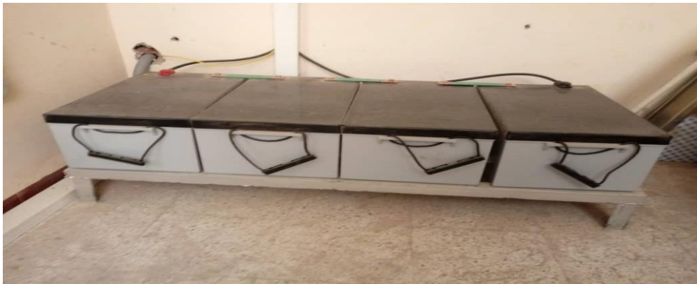
Figure III.12 : Emplacement des batteries.
