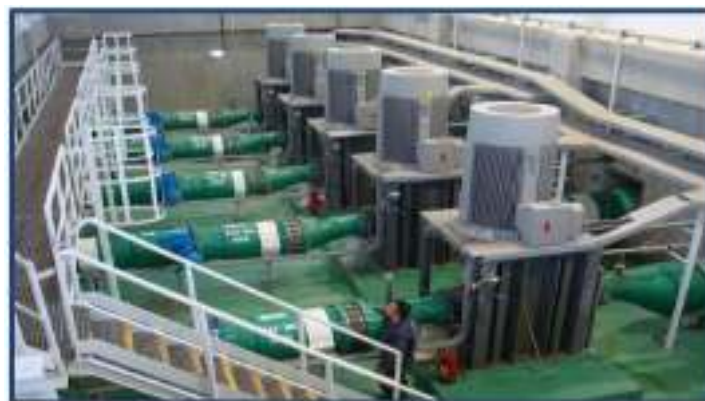
Figure III.3: station de pompage de l'eau de mer
