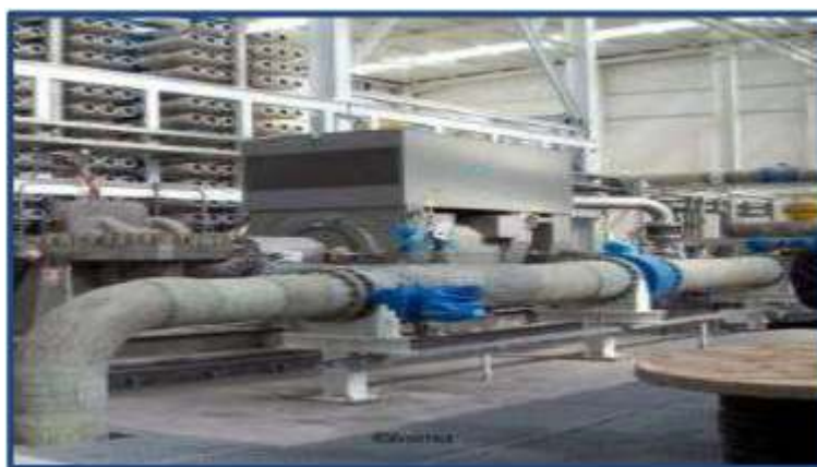
Figure III.7: pompe à haute pression.
