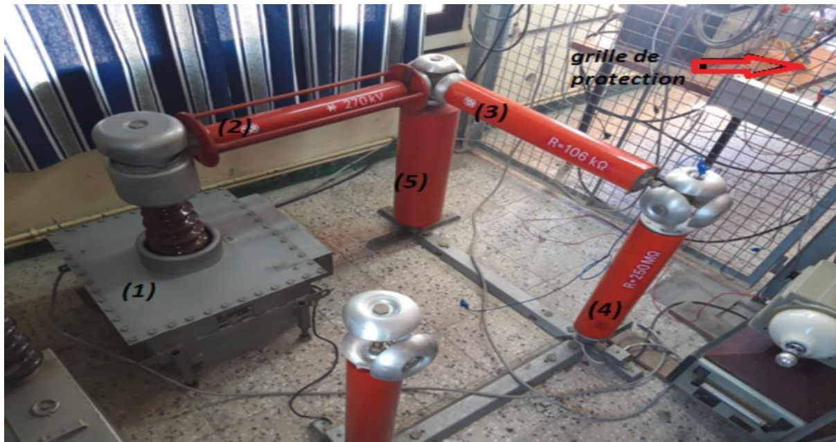
Fig II.8 : Installation de haute tension
