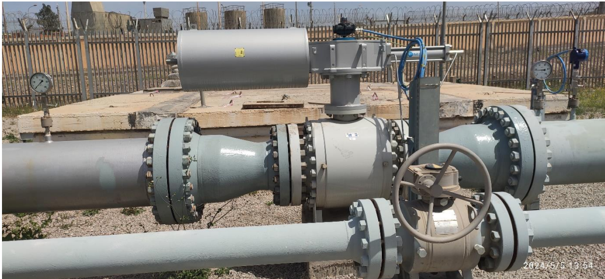
Figure I.5 : La vanne PCV de la station SBM.
