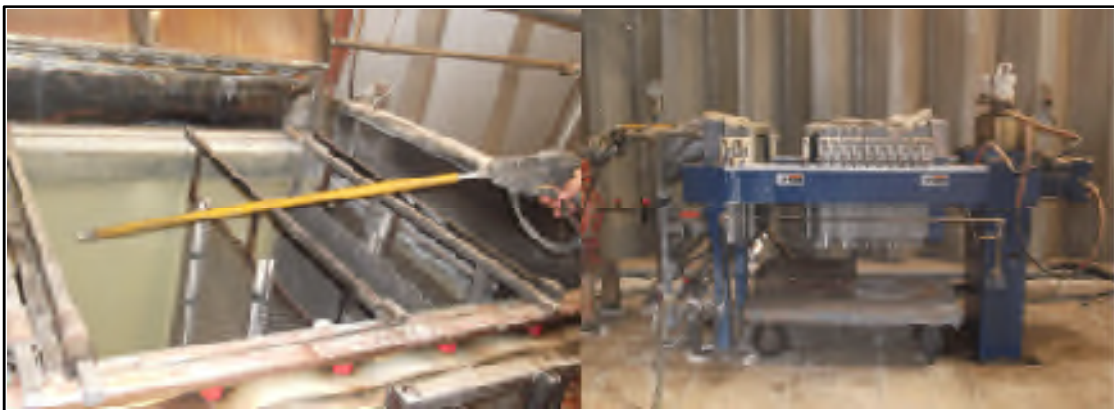
Figure II.9: Cellules d'élution et filtre presse.[Source: Photo prise]
